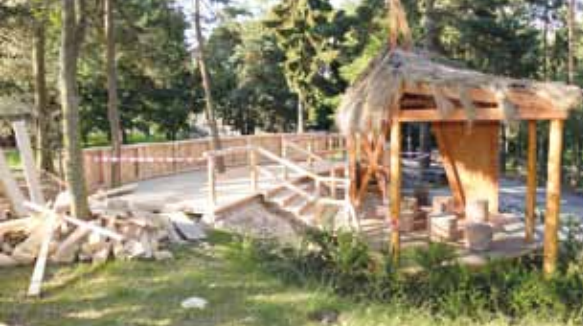
Stavba vyhlídky v Safari Afrika /The construction of a observation point in the African safari/
