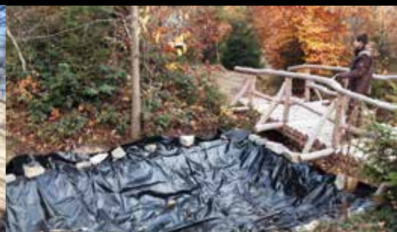
Položená folie na jedné z tůní /The laid plastic film on one of the water pool/
