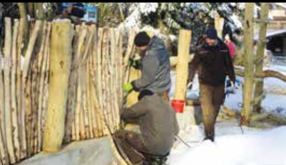
Plot u výběhu koz zakrslych /The fence in the paddock of dwarf goats/
